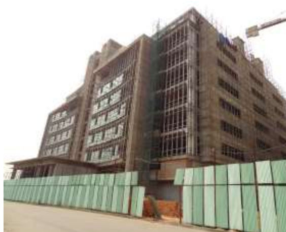
BUILDING HAD BEEN BARRICADED
