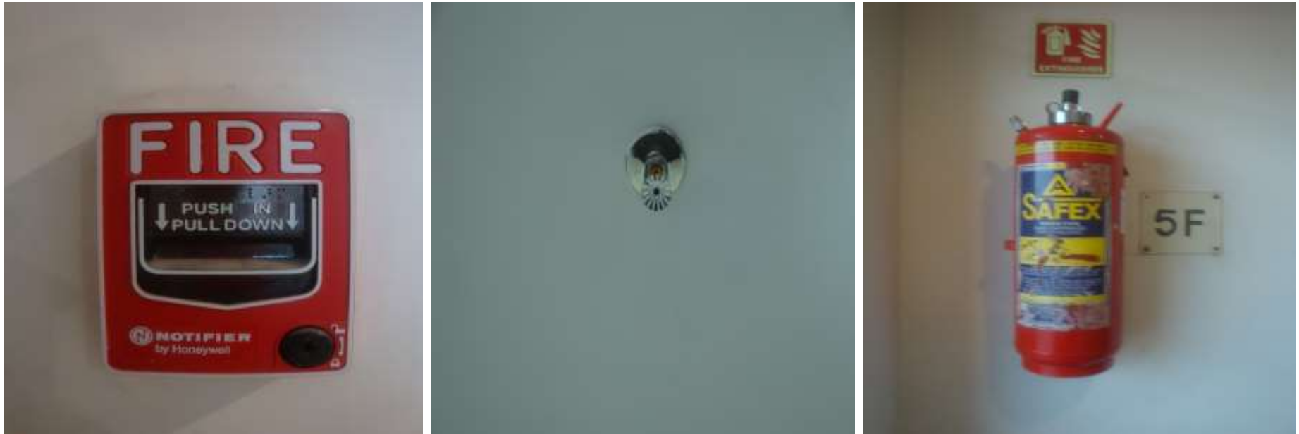
FIRE FIGHTING SYSTEM
